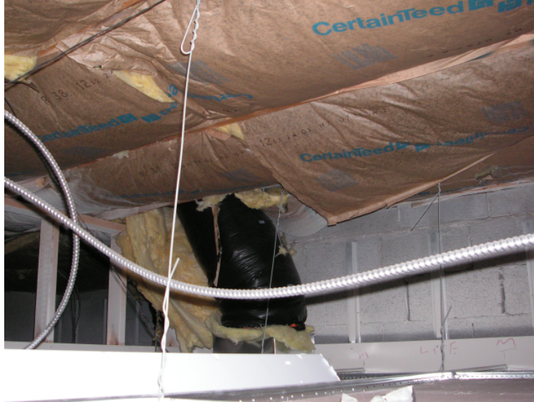
Photo - 5: Complete absence of an air barrier on the underside of the roof trusses allows for excessively high exfiltration and infiltration. Also without support the insulation will fall out. Flexible ducts should not penetrate insulation.
