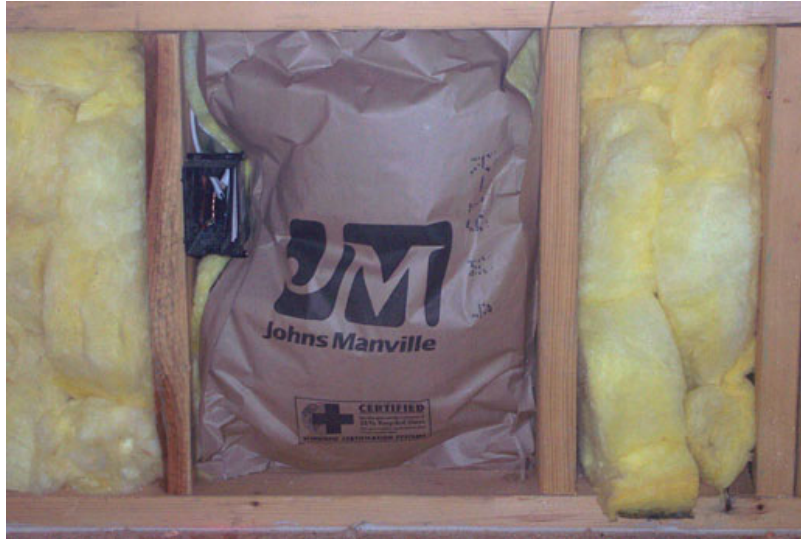
Photo – 1: This is an example of compressed insulation, improperly fit around an obstruction, and within the cavity. The overall effectiveness of this insulation is greatly reduced.
