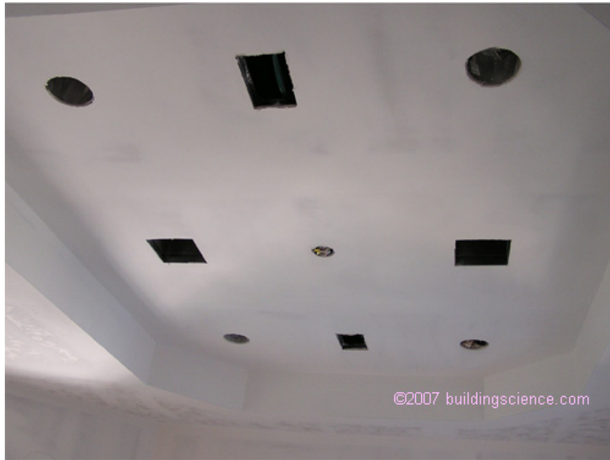
Photo – 3: Penetrations of the air barrier allow for high infiltration or exfiltration ( air movement between the conditioned space and attic).
