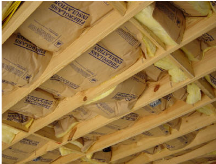
Photo – 2: Poorly installed insulation in the ceiling.
