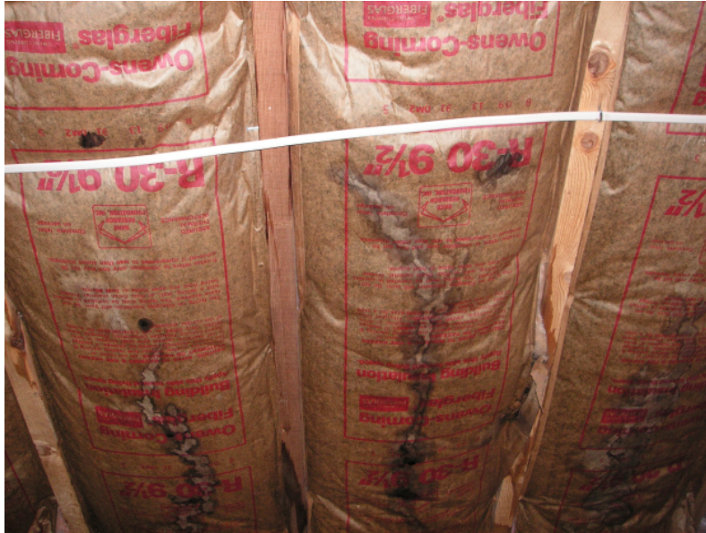
Photo – 7: Water stains are from condensation forming on the underside of the roof deck.
